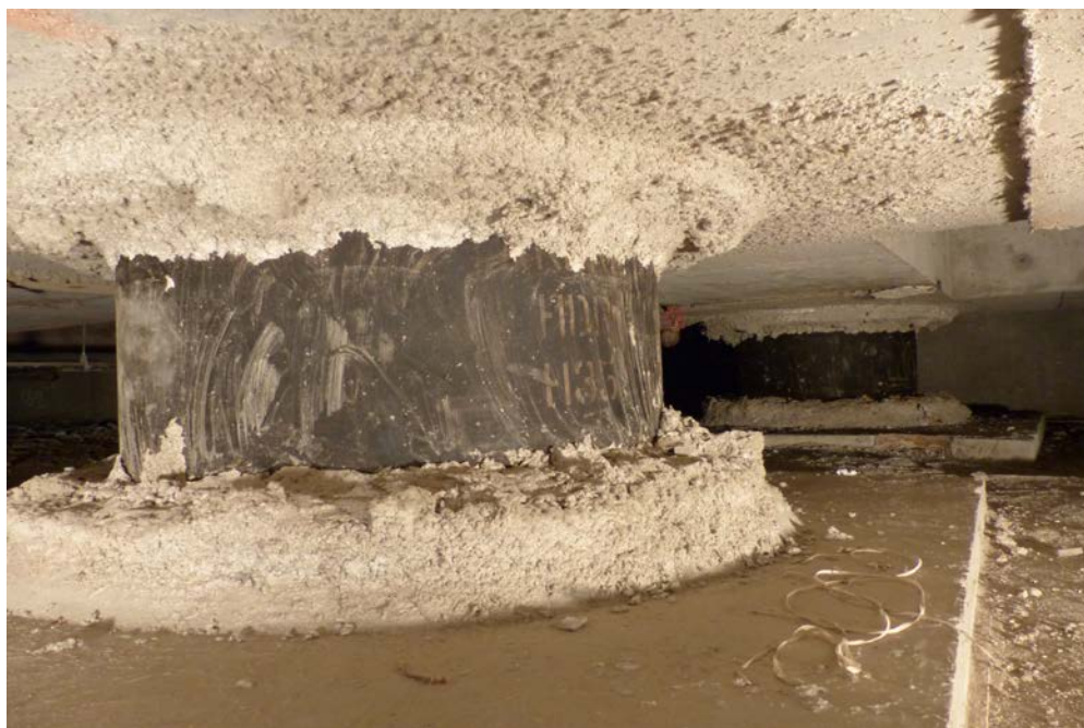
Fig. 1.4: A total of 134 base isolators in the subbasement of the Hearst Memorial Mining Building, like the two shown here, keep the floor of the building (above) seismically separated from the ground (below).
