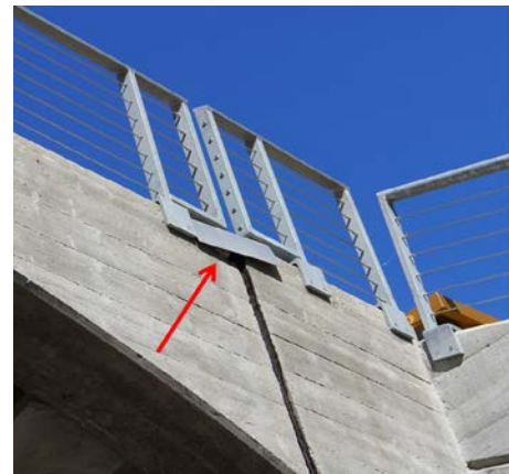
Fig. 5.9: Movement due to fault creep in the arch of the north tunnel
