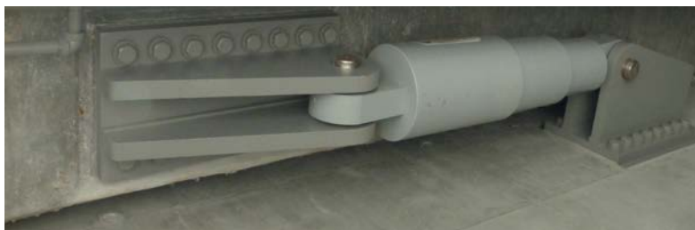
Fig. 5.14: In order to reduce the overall level of shaking between the various sections of the stadium and the press box, they are connected by massive hydraulic dampers.
