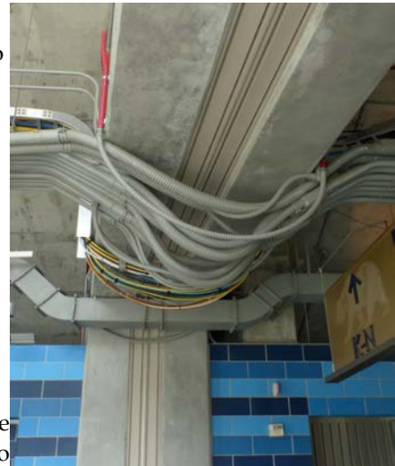
Fig. 5.13: Flexible conduits were installed to reduce the chance that lifelines rupture during an earthquake. Note the plastic cover separating two separate sections of the stadium.
