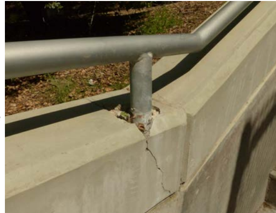
Fig. 5.6: Cracks in the handrail support
