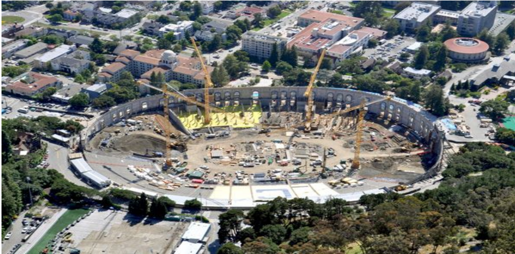
Fig. 5.4: During the renovation from 2010 to 2012 the stadium was entirely gutted except for the exterior wall. This aerial view from the east is looking over the stadium towards campus. When this picture was taken the construction of the new press box had not yet commenced.
