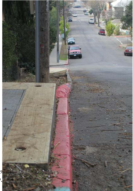
Fig. 7.1: Street curb offset by aseismic creep looking west down Dwight Way.
