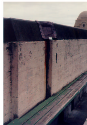
A. Right-lateral displacement of stadium parapet at expansion joint between Sections K-KK (south end of stadium).
