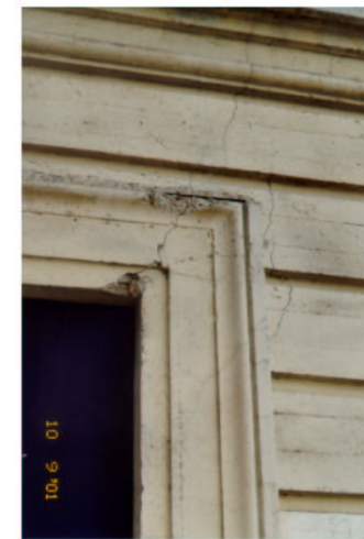
B. Cracking at corner of entryway to stadium in Section A (north side of stadium).
