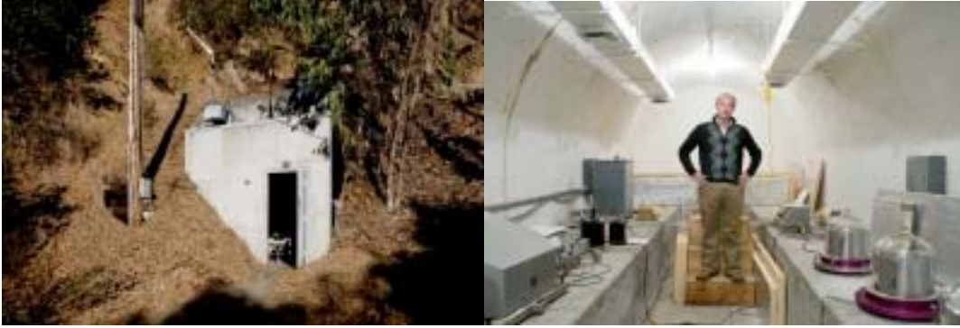
This Cold War–era vault in the Berkeley Hills was built to listen for Soviet nuclear tests; now its sensitive equipment listens for earthquakes.
